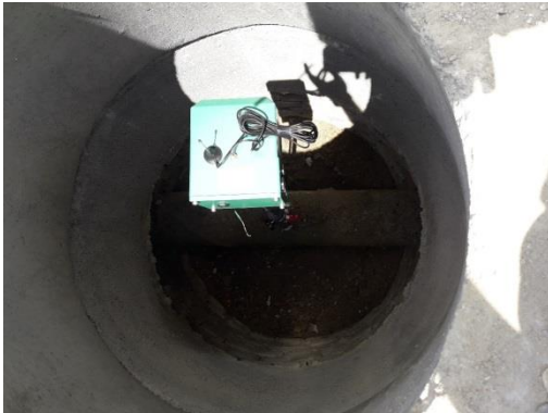
Figure 3.5.1 – manhole with insertion flow meter at the entrance of DMA Dunav
