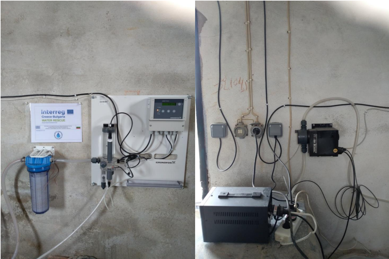
Figure 3. Chlorination devices installed
