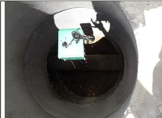
Picture 1 – manhole with insertion flow meter at the entrance of DMA Dunav
