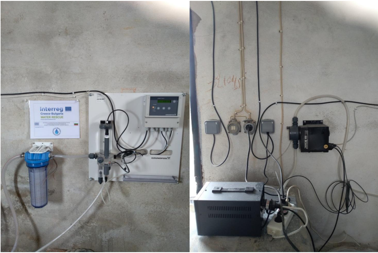
Figure 3.2.3. Chlorination devices installed
