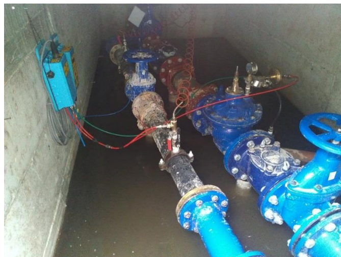
Figure 23. PRV installed in a water distribution network (Kanakoudis & Tsitsifli, 2015)
