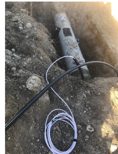
Ultrasonic flowmeters installation
