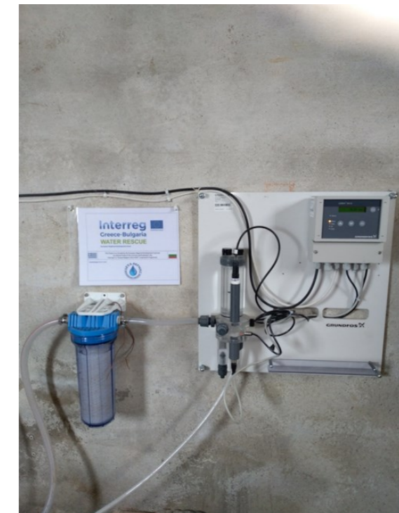
Chlorination device installed
