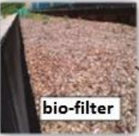
liquid waste tanks
