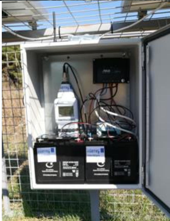
Figure 9. Environmental Measurements Station 3
