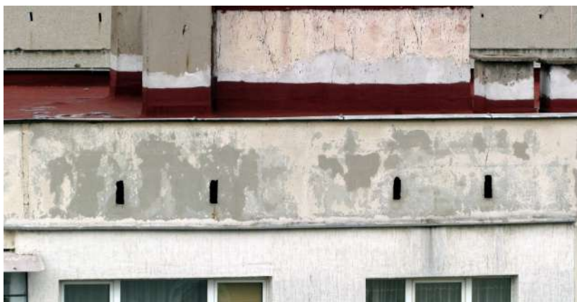
Cracks on facades of buildings that are easily available from the bats
