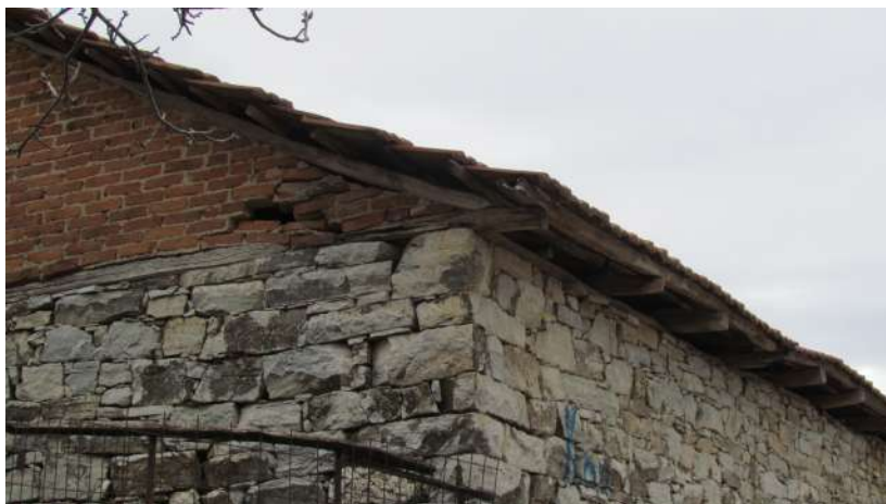
Suitable opening for bats to go inside in attic of old house
