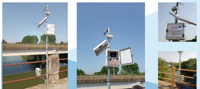
Main components of a Floodguard river monitoring station
