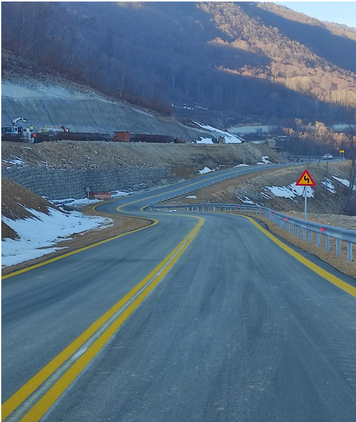
Photo 1: Deviation in Cut O20 (ch. 13+300,00 – ch.13+690,00)
